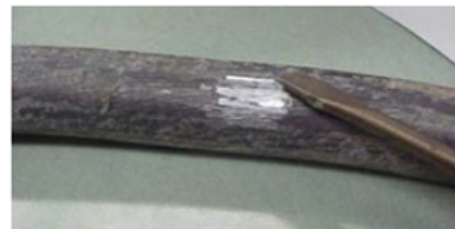
Lead Piping Example
